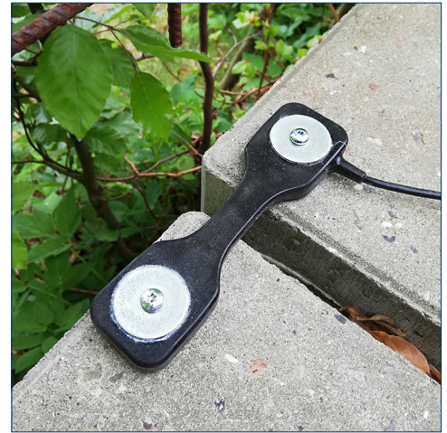
Structural Deformation: Monitoring rate of deformation caused by foundation settlement.
